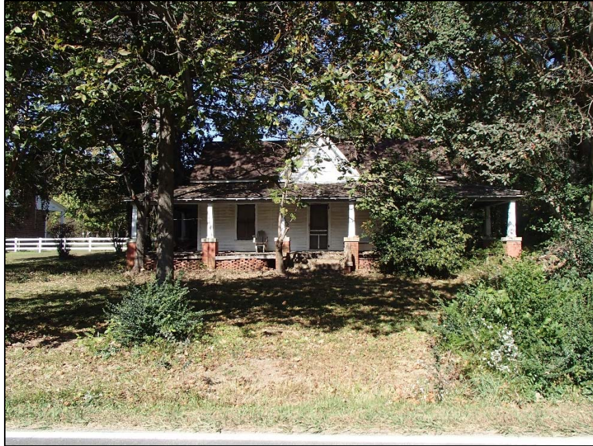
Figure 18: Rougemont tri-gable, Red Mountain Road, unaltered except for a later but historic porch
